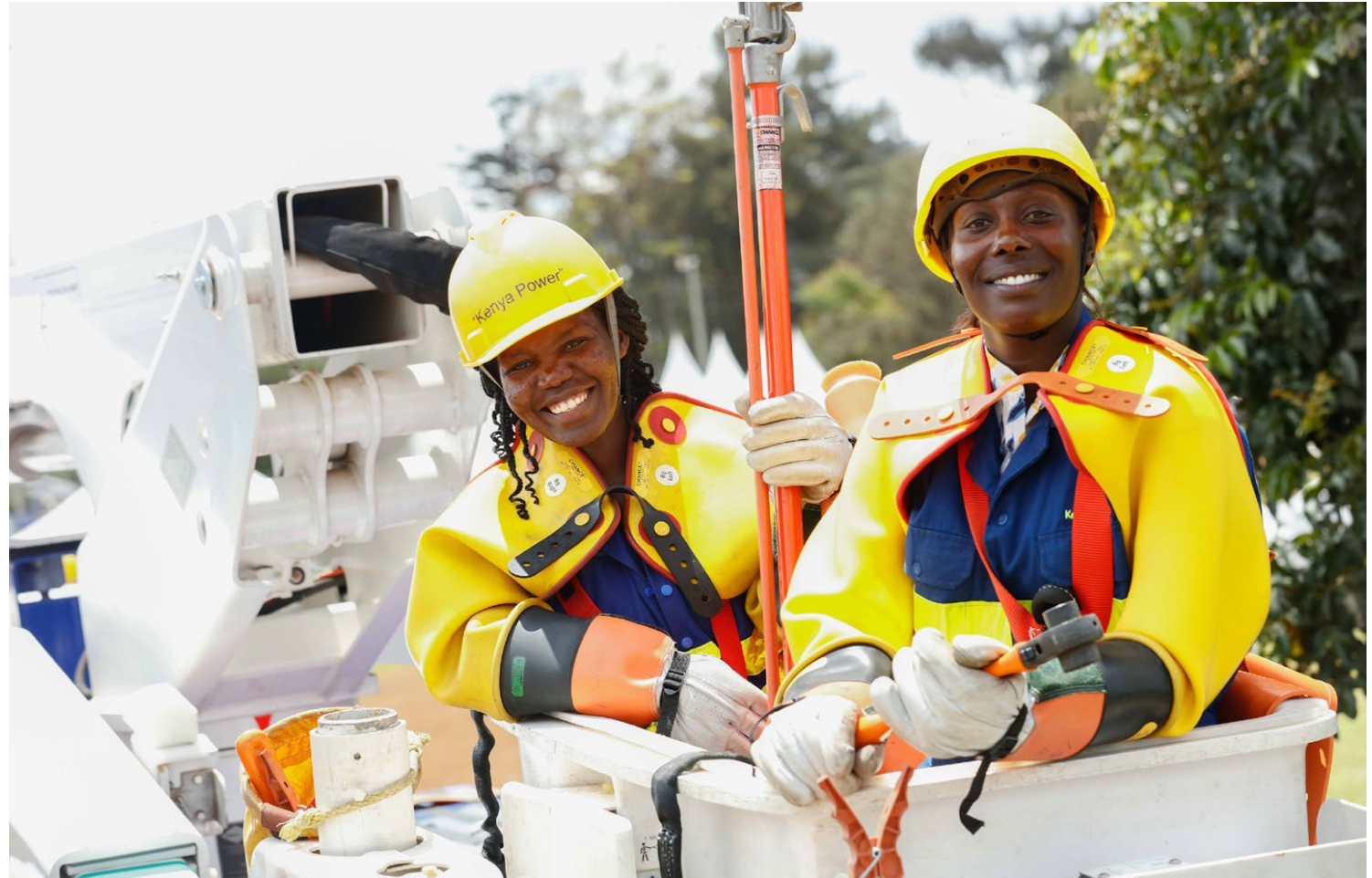
Two female power line workers implement KPLC Kenya's live line maintenance program to reduce power outages.
